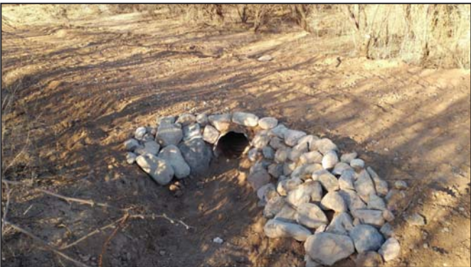
To level the trail for handicap-accessibility, four culverts needed to be constructed along the trail. These washes had water flow during last year's monsoons.
