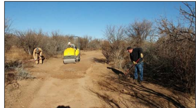
Before the trail material is laid down, the soil must be compacted with a rented roller.
